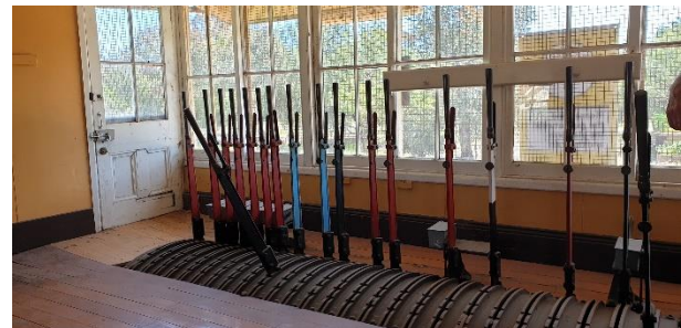
Inside the Signal Box at Avenel Railway Station
